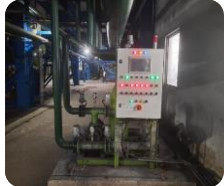
Condenser on-load cleaning system
